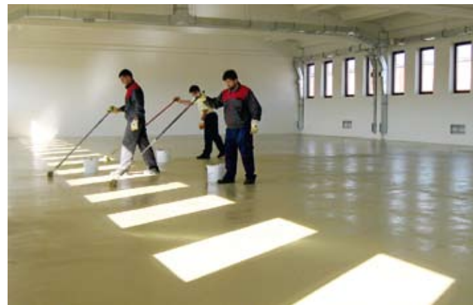
TELEKOM SRBIJA - KRALJEVO BRANCH, EPOSAN E (550m 2 )
